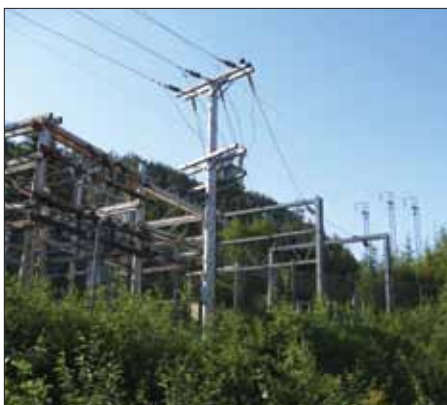
Existing substation at Kitsault Mine
